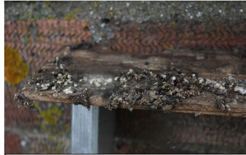
The bat box at Conington Mill pumping station was used by bats in 2017 and in early May 2018 when both bat droppings and signs of roosting birds were present.
